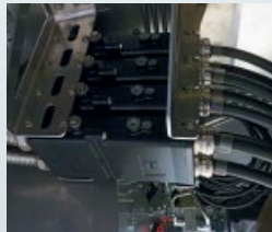
power connection for thruster
